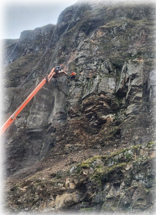
Hanging rockfall protection mesh at Stepped Cut
