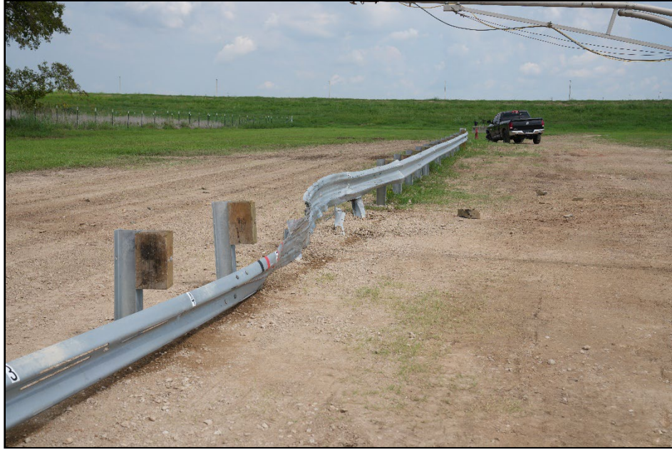
Figure 8.5. TL-2 W-beam End Terminal after Test at Impact Location 615181-01-5.
