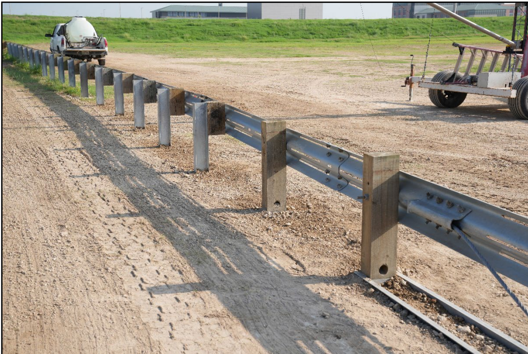
Figure 5.7. Field Side of the TL-2 W-beam End Terminal Installation prior to Test 615181-01-5.
