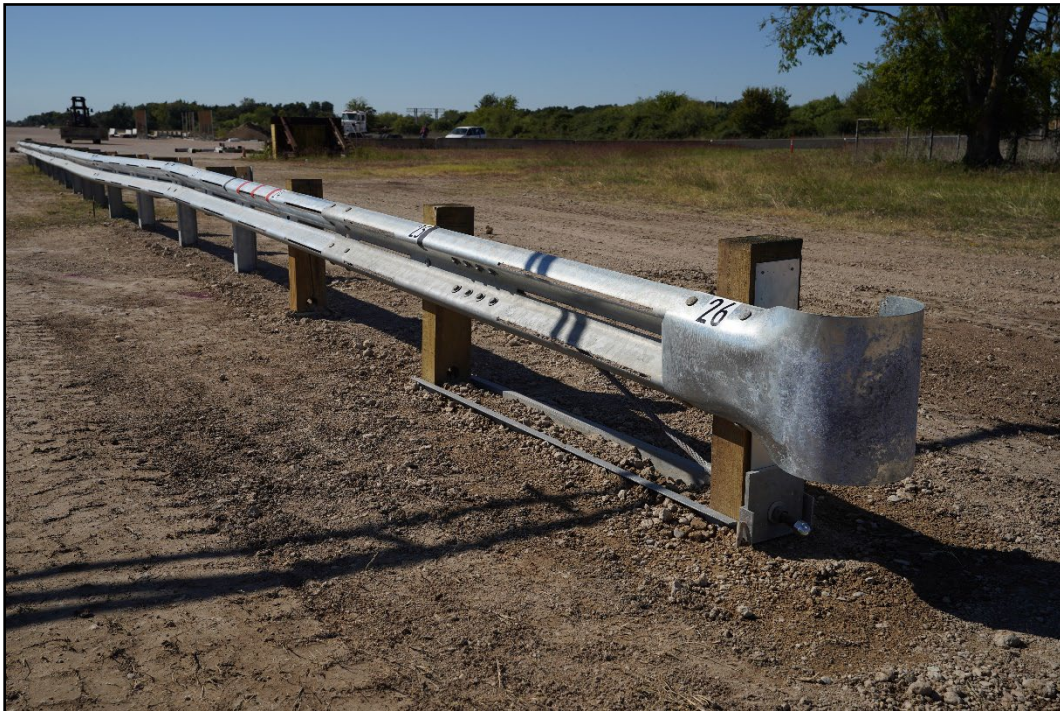
Figure 5.17. Downstream View of the TL-2 W-beam End Terminal Prior to Test 615181-01-13.
