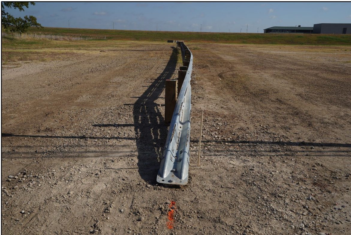
Figure 3.32. In-Line View of the TL-2 Terminal on MGS prior to Crash Test 615181-01-3.
