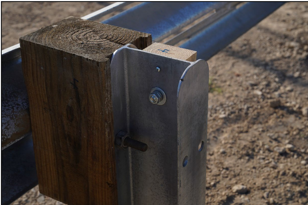
Figure 5.12. TL-2 W-beam End Terminal on the Non-Impact Side of Post 4 prior to Tests 615181-01-11 & 615181-01-12.
