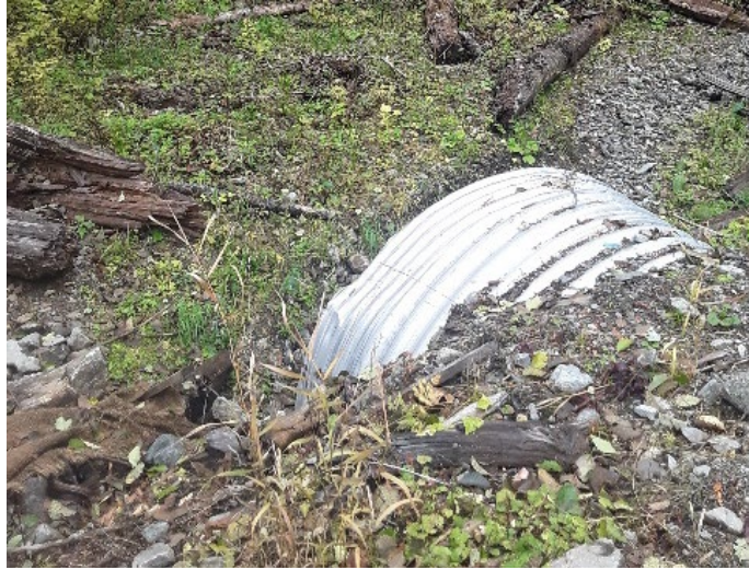
Figure 3-9: Storm Damage in North Cascades National Park
