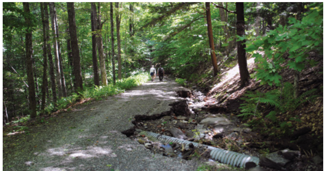
Damage caused by Tropical Storm Irene at Marsh-Billings-Rockefeller NHP in 2011. Photo by NPS.
