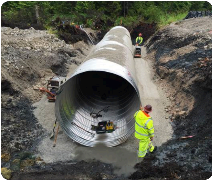
The first of four installed on the project, this 108 inch AOP replaces a 36 inch culvert
