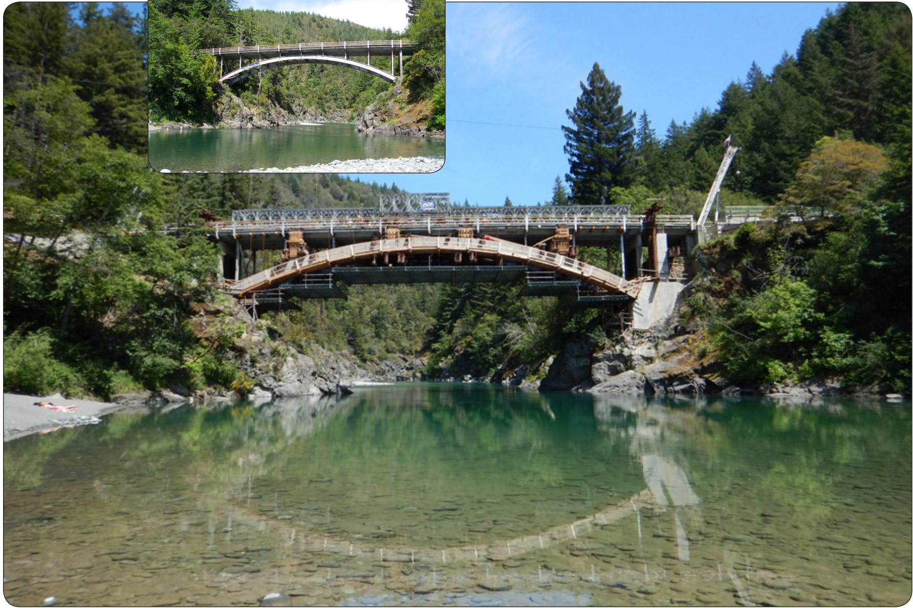
Replacement of the historic South Fork Smith River Bridge. Work continues through staged construction, under a CMGC contract. The main arch is undergoing reconstruction with the original bridge still in place and carrying traffic during construction. — Crescent City, California
