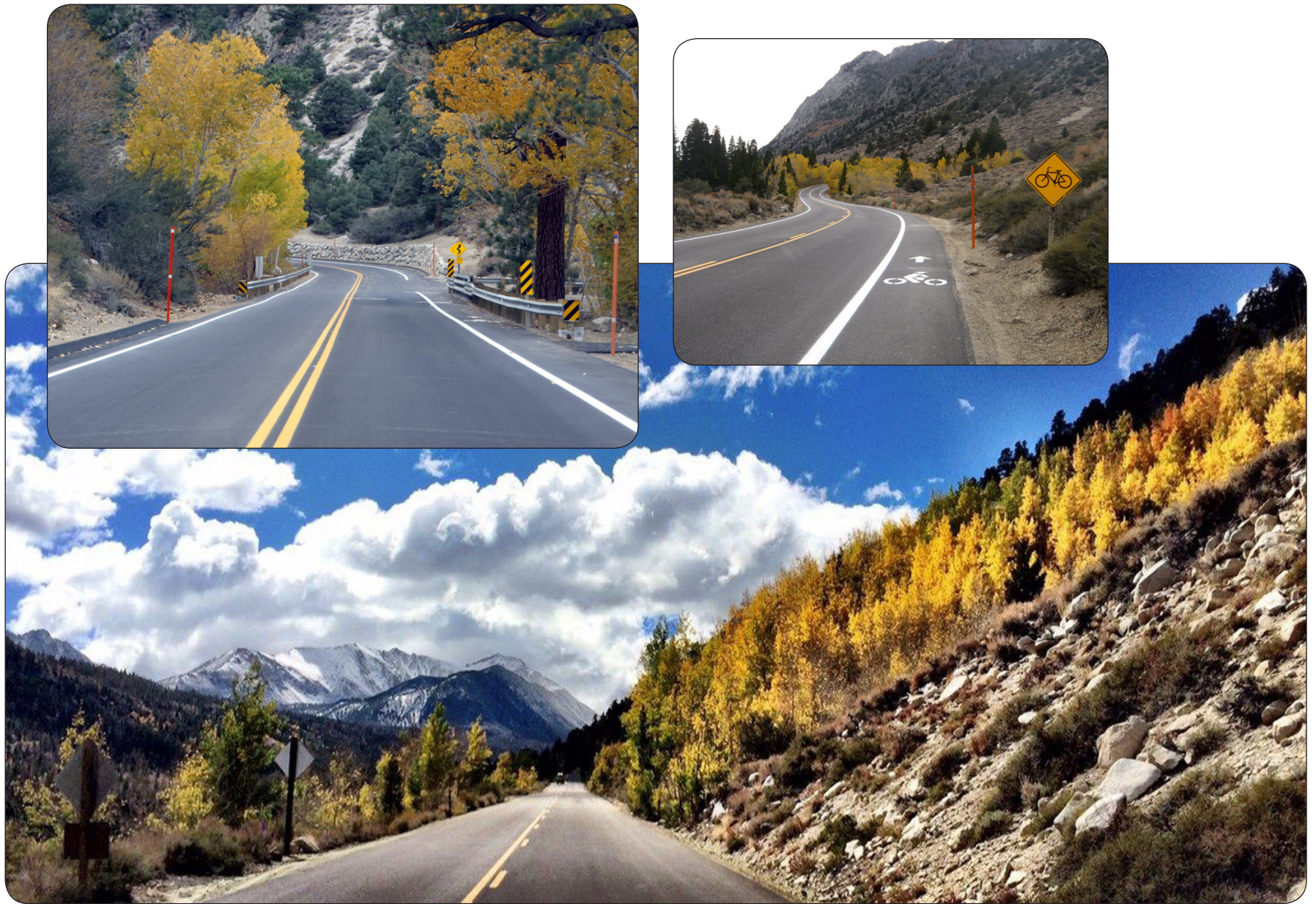
Reconstruction and rehabilitation of Rock Creek Road included widening to accommodate shared use shoulders, (insets) this necessitated use of rockery and MSE walls to accommodate widening. — Forest Highway 89, Inyo National Forest, California
