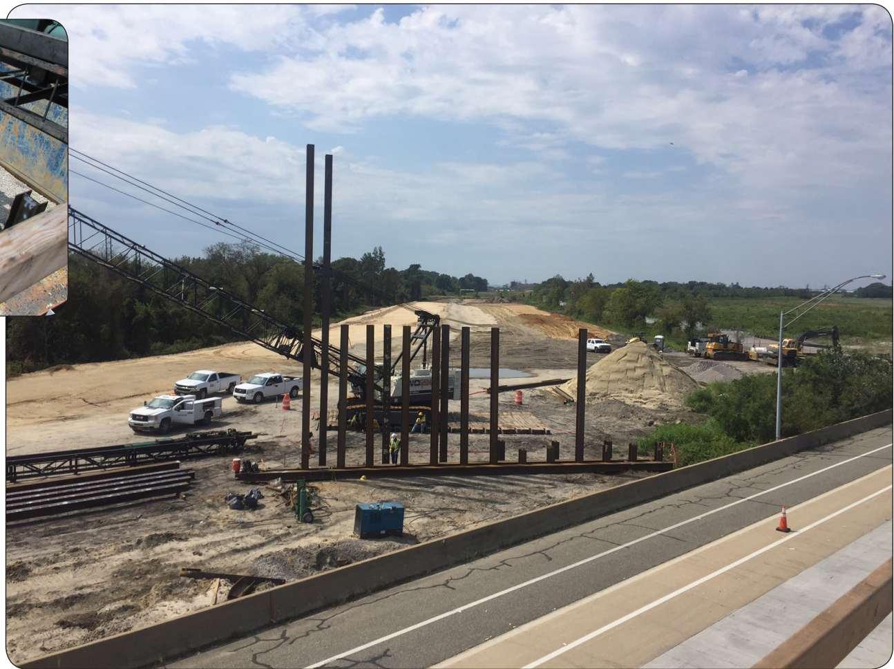
I-564 Ramp C Flyover Bridge construction looking West to Hampton Boulevard Norfolk International Terminals North Gate, the Virginia Port Authority's largest terminal, Norfolk, Virginia
