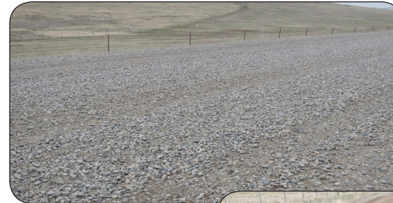
Untreated road constructed in 2012 Note: raveling, loose surface condition, aggregate loss
