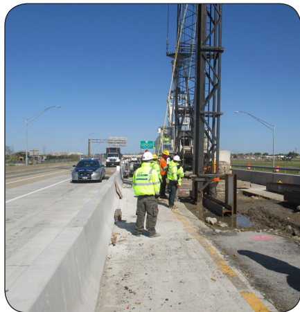
Driving production pile in Pier 1A foundation for the Ramp C Flyover Bridge 602
