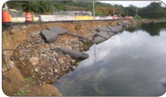
Damaged Roadway embankment
