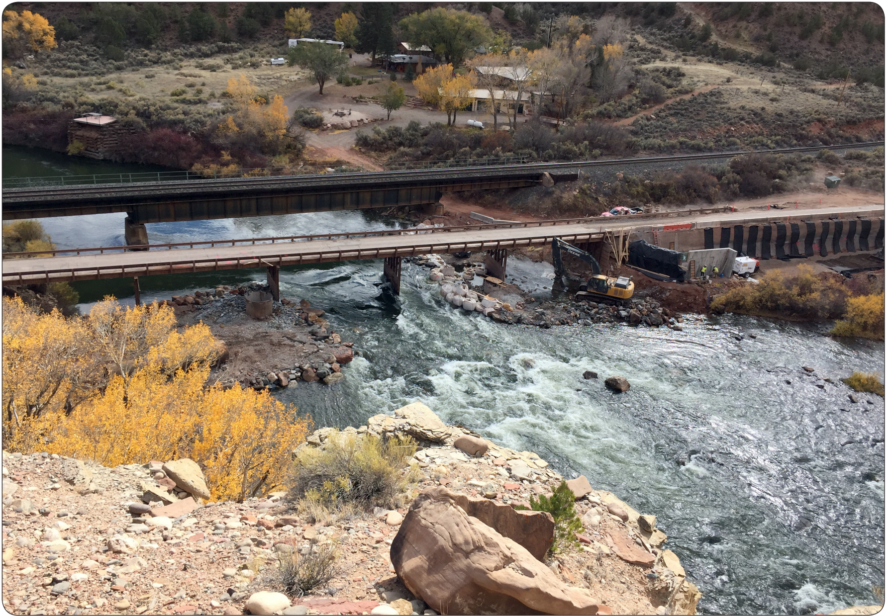
Red Dirt Bridge constructed in 1945 spans the Colorado River, the existing 200 foot long 5-span steel bridge (foreground) running parallel with a railroad bridge is undergoing replacement under the FLAP program. — Colorado River Road, Gypsum, Colorado
