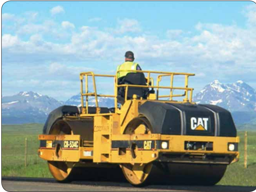
Blackfeet Tribe paving project — Tribal personnel operating breakdown roller from the Rocky Mountain Region's equipment pool
